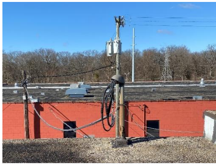
Figure D-62: Utility pole, transformer and weather head
