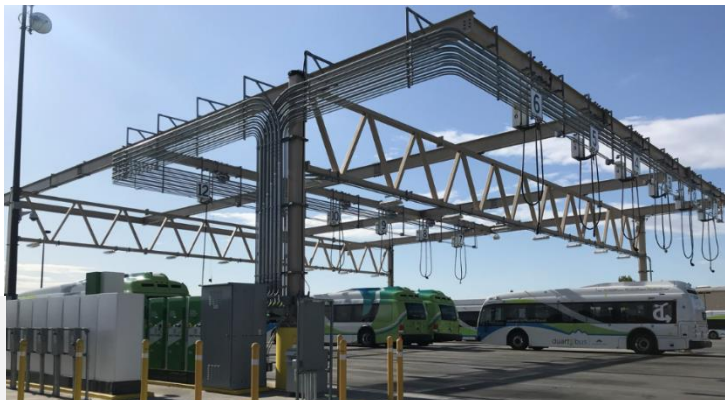
Figure D-67: Example of plug-in charging with overhead mount chargers at Foothill Transit in San Gabriel and Pomona valleys, CA
