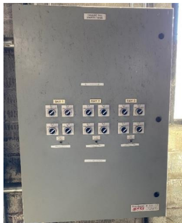
Figure D-65: Typical panelboard
