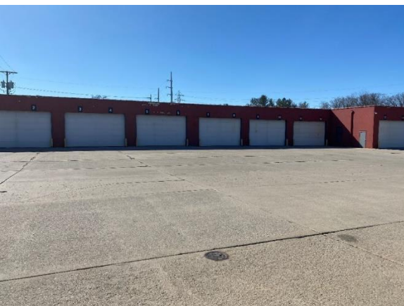
Figure D-3: North of the storage barn, general condition of pavement.
