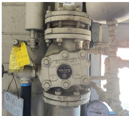
Figure D-54: Fire water service entry
