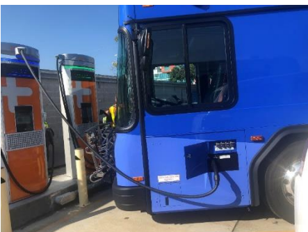
Figure D-67: Example of plug-in charging ground chargers at Big Blue Bus of Santa Monica, CA
