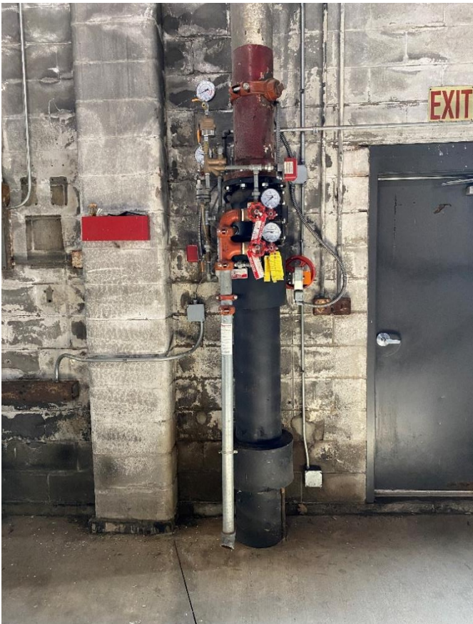
Figure D-56: Fire water service entry
