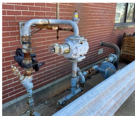
Figure D-55: NIPSCO natural gas entry
