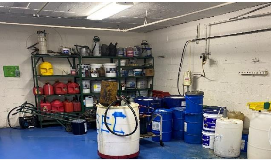
Figure D-32: Valve room
