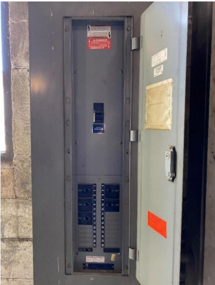
Figure D-63: Service entry panel
