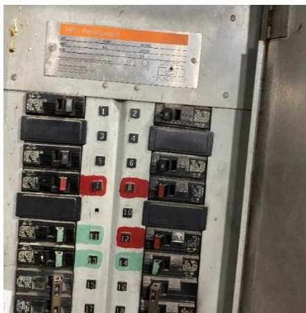
Figure D-64: Typical panelboard
