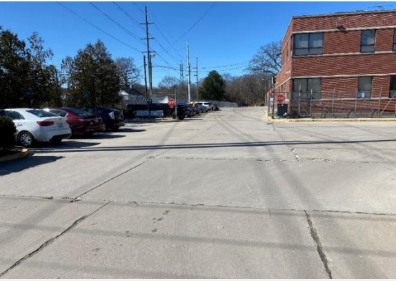
Figure D-2: South entrance looking west, general condition of pavement.
