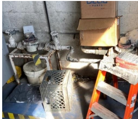
Figure D-53: Water service entry in service
