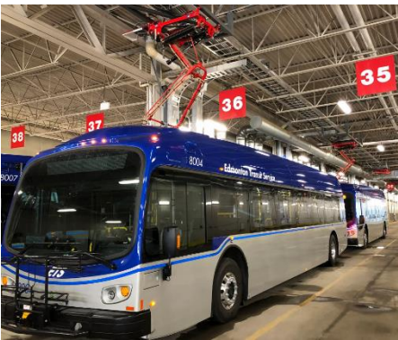
Figure D-66: Example of in-depot pantograph charging system at Edmonton, Canada
