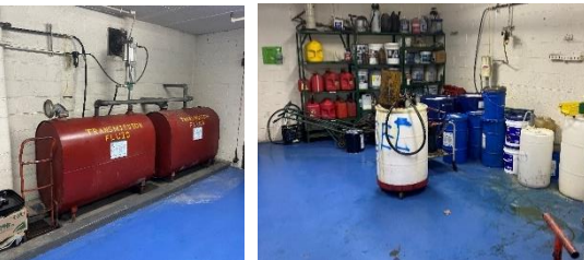
Figure D-52: Fluid storage tank room
