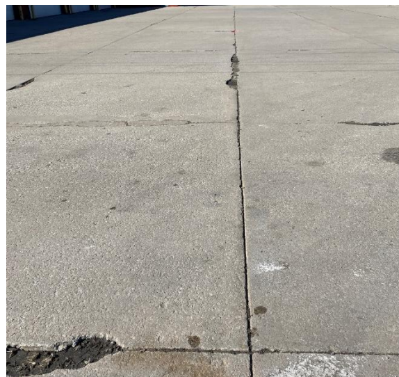
Figure D-4: Photo north of the Storage Barn, general condition of pavement.
