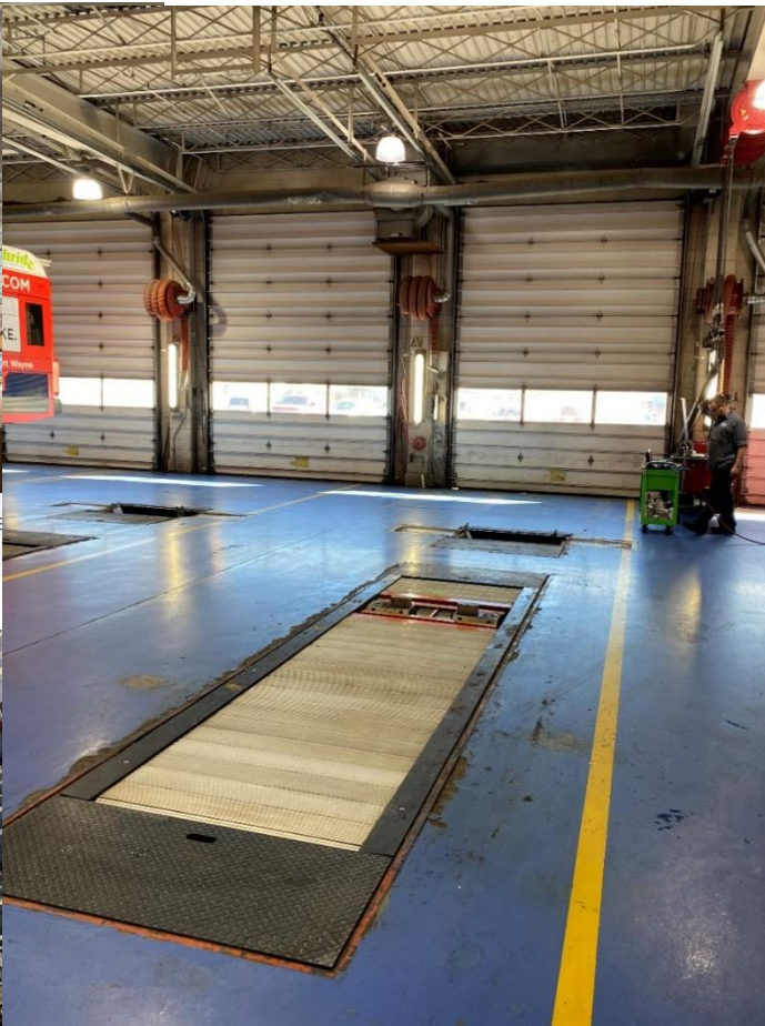
Figure D-12: Typical floor slab condition.
