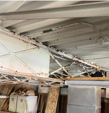
Figure D-10: Corrosion developed at the base of column.
